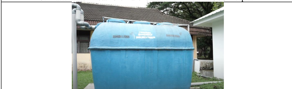
4. Waste Water Treatment Plant at USU Dental and Oral Hospital
