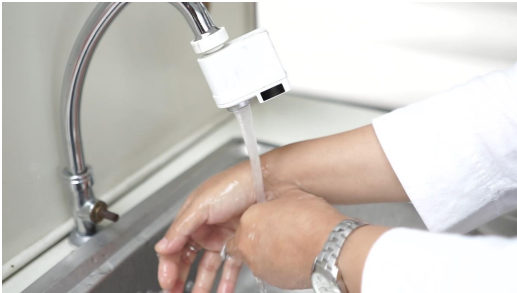
Sensor-activated Faucets in the Central Administrative Building
