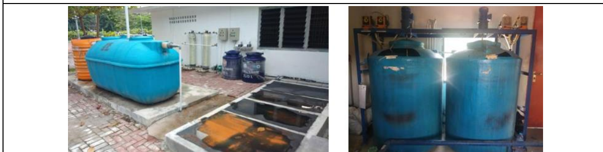
Wastewater Treatment Plant in the Isolation Room of USU Teaching Hospital
