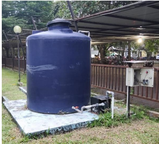
Rainwater Harvesting near the Central Administrative Office Building
