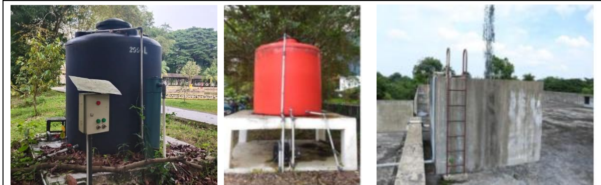
Rainwater Harvesting at the Faculty of Engineering
