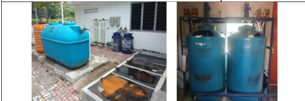
3. Waste Water Treatment Plant for Isolation Room at USU Hospital
