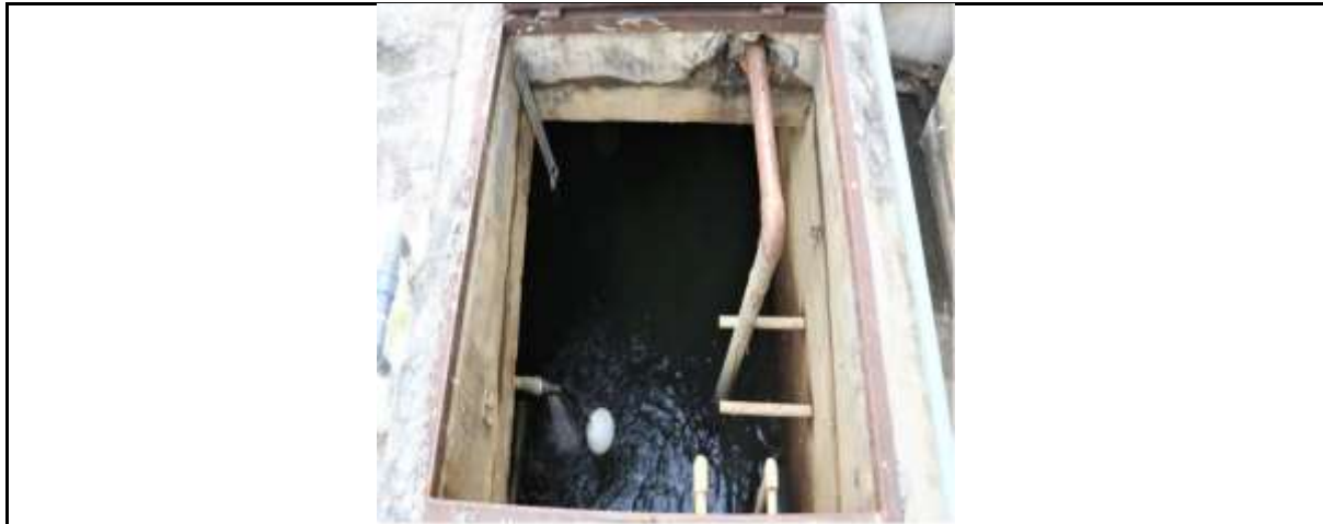
Use of Water Tanks Equipped with Balls (Automatic Buoys) at the USU School of Public Health
