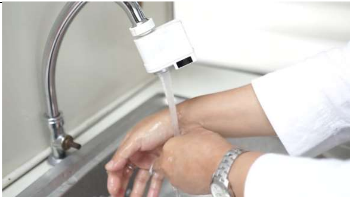
Sensor Water Faucet in Central Administration Building
